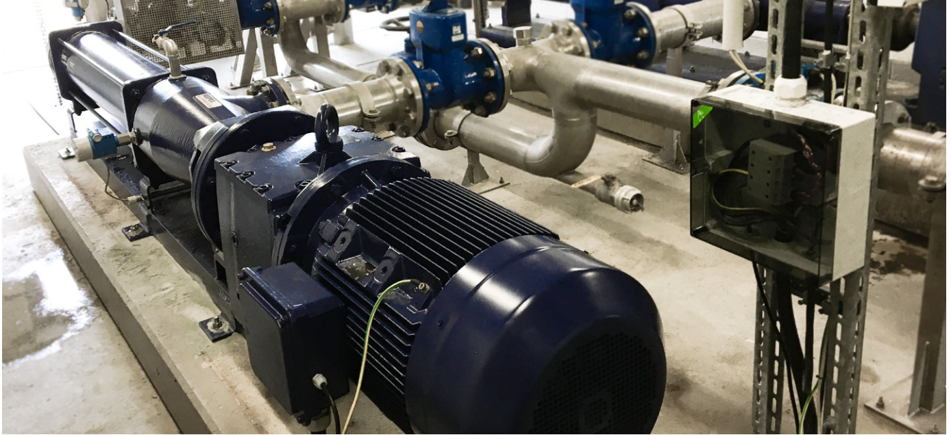
SEEPEX Pump Monitoring at the WWTP in Essen-South.
